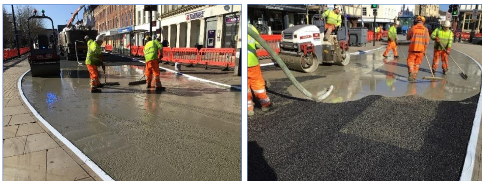
In areas subject to heavy loading and stresses materials such as grouted asphalt can be used for a more durable surface.
