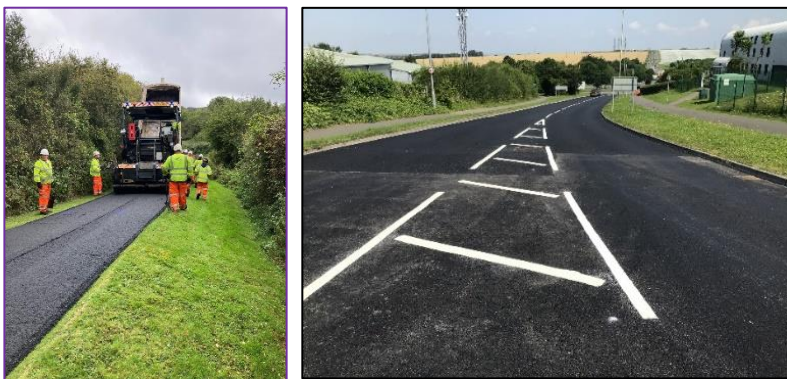
Resurfacing, often with the existing damaged surface being removed, produces a durable surface and is used where the underlying construction is suitable.
